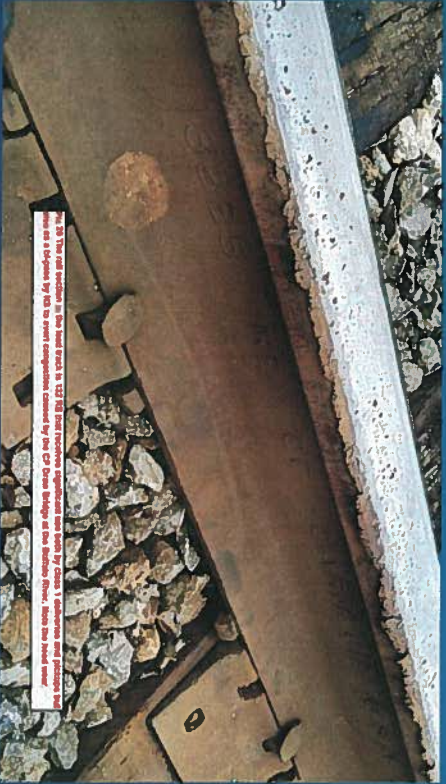
19 Existing track at Lockwood Products shown from the east looking up the track.
