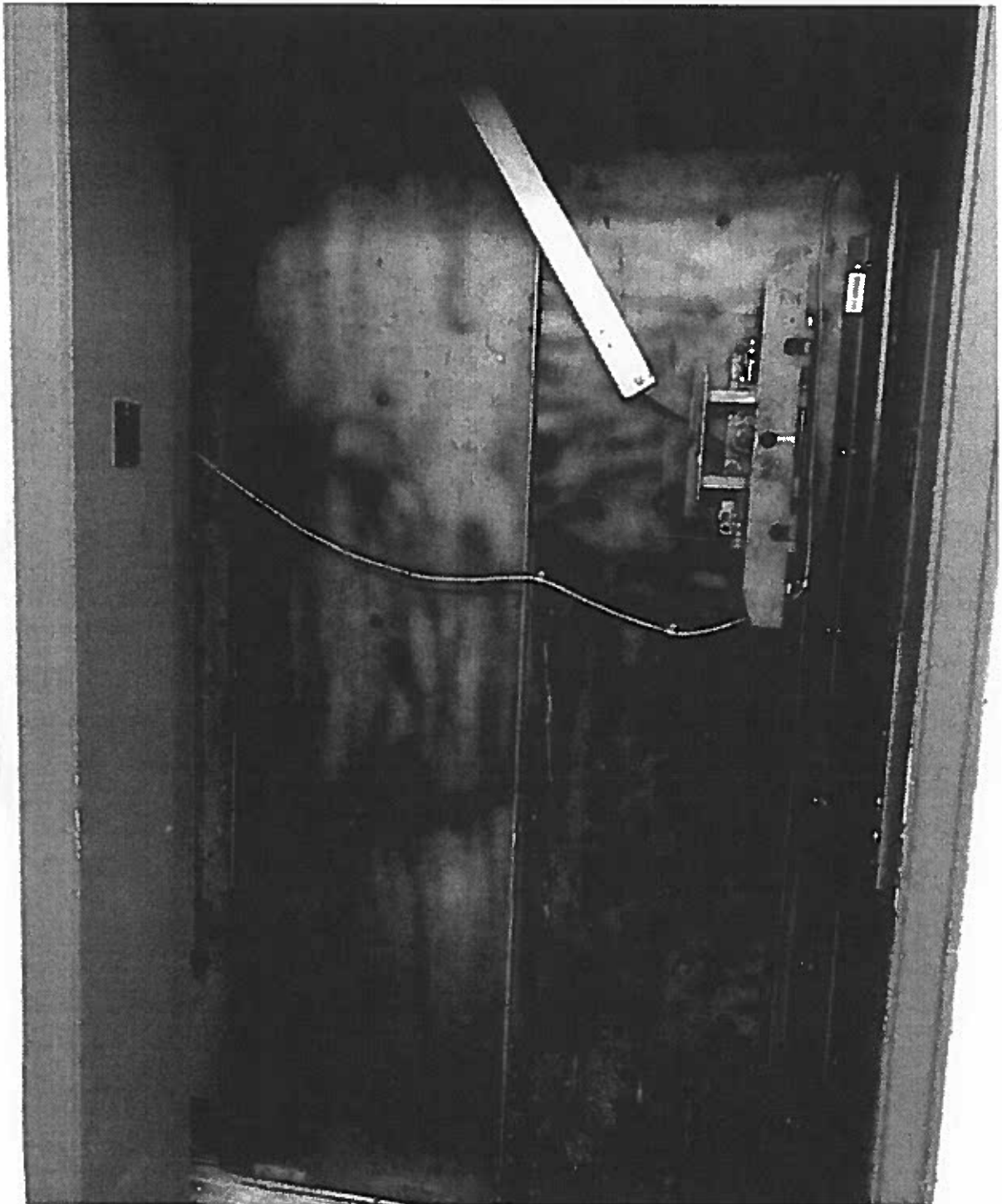
Brooklyn College, Broken Elevator
